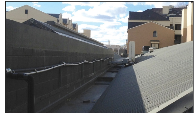
Service infrastructure (above) located on roofs (antennae, communication structures, air conditioning units, satellite dishes, etc.) should be hidden behind parapet walls and roof structures.
