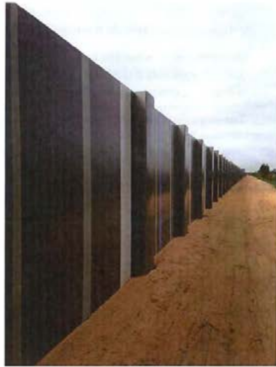
Plate 18 Acoustic wall likely to be installed adjacent to north-west boundary of the site, approximately 3m high with 3m-wide firebreak
