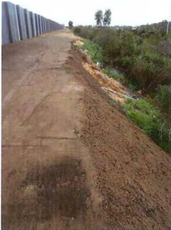
Plate 17: Acoustic wall installed in the northern portion of Lot 9001 Mortimer Road, adjacent to the Kwinana Freeway showing firebreak and interface with vegetation.
