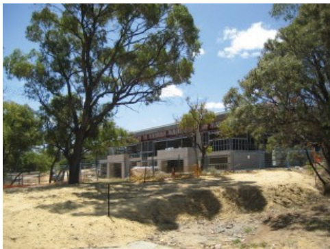
The TAFE facility under construction on the corner of Gilmore and Sulphur Avenues
